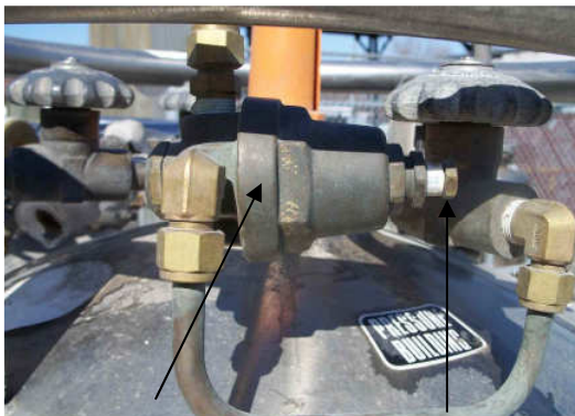
Pressure Building Regulator
